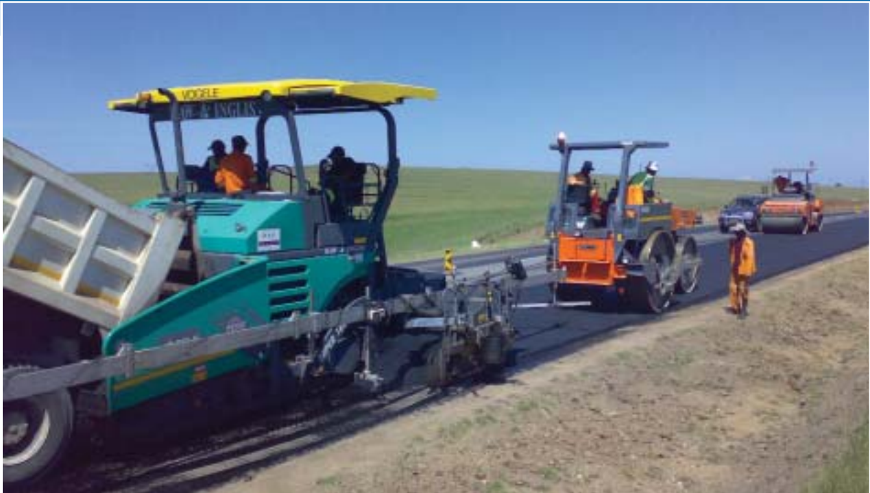
Paving of bitumen treated base course in progress on the N2 Mthatha to Nqadu Forest rehabilitation project in the Eastern Cape.
