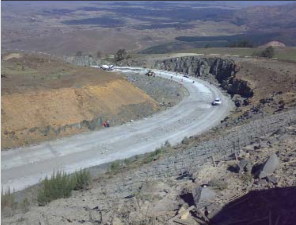
A blast cut on the new road from Langeni to the R61.
